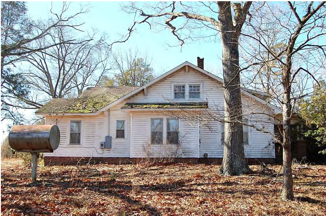
William T. and Doris W. Redwine Farm, House, Side (East) Elevation, Looking West.
