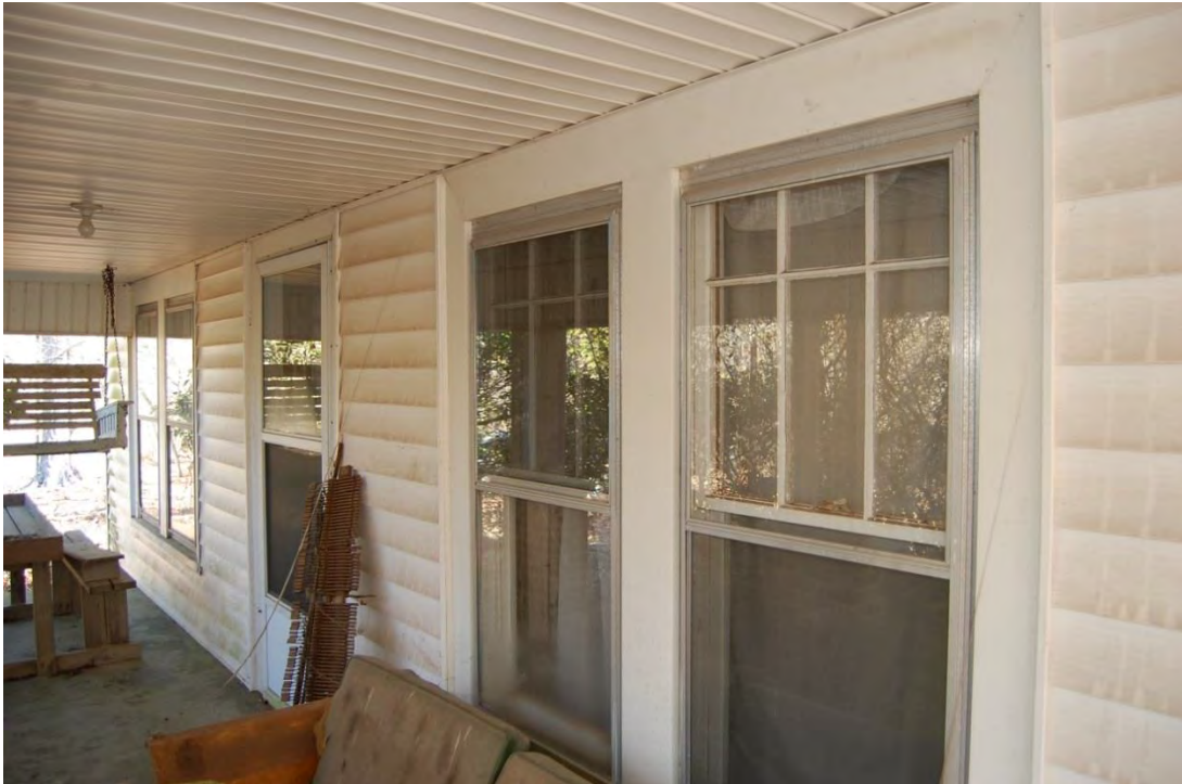
William T. and Doris W. Redwine Farm, House, Façade, Looking East Along Front Porch.
